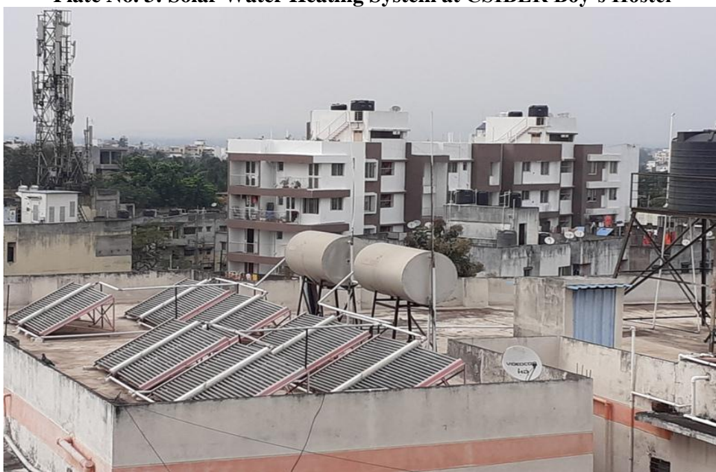
Plate No.4: Solar Water Heating System at CSIBER Girls Hostel
