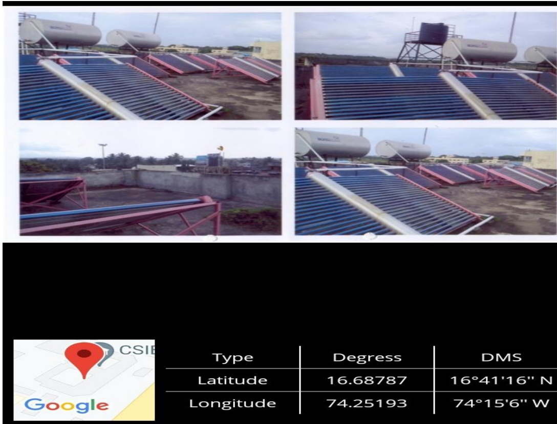
Plate No. 3: Solar Water Heating System at CSIBER Boy's Hostel
